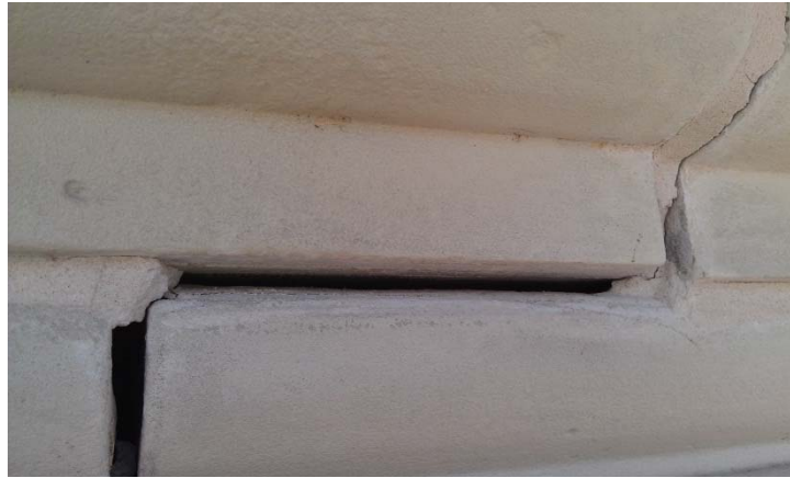
Figure 22. Exterior stone cornice separation.
