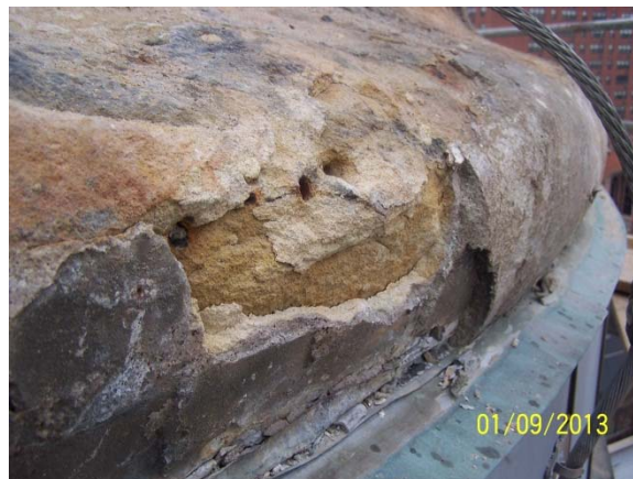
Figure 25. Exterior bell tower dome cementitious repairs distress.
