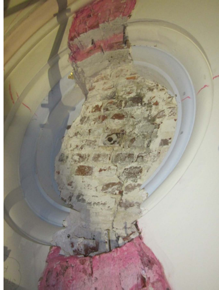
Figure 24. Cracking and plaster repair at main dome coffers.
