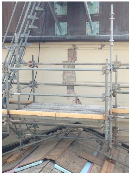
Figure 14. Exterior through-wall crack above brick masonry arch.
