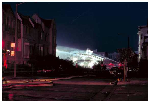
Figure 4. Demolition of collapsed building and watering down of burned area, October 18, 1989, Beach and Divisadero Streets, Marina District after the October 17, 1989, Loma Prieta CA Earthquake (C.E. Meyer, U.S. Geological Survey).
