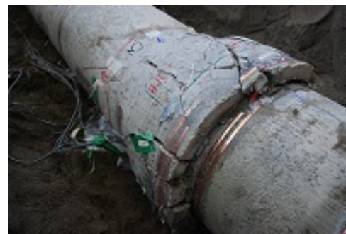
Figure 5. Damage detection and health monitoring of buried pipelines ongoing NEESR project conducted at the NEES@Cornell Equipment Site by University of Michigan (Prof. R. Michalowski, PI), and researchers from Purdue University, Virginia Tech, and Merrimack College).
