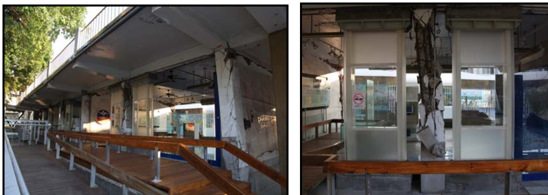
Figure 1. The Damaged South Classroom in 921 Earthquake Museum of Taiwan (Left: View from northwest; Right: AW retrofit)
