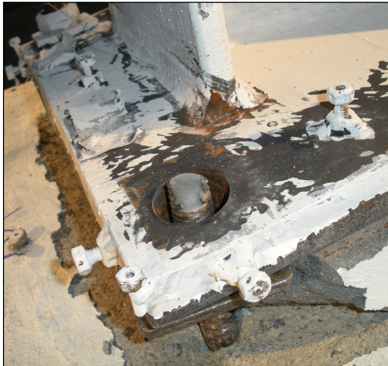
Figure 3.23 – Fracture of anchor rod from Test #2
