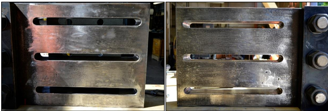
Figure 4.100: Condition of the internal steel plate surfaces at the beginning of Phase II-3
