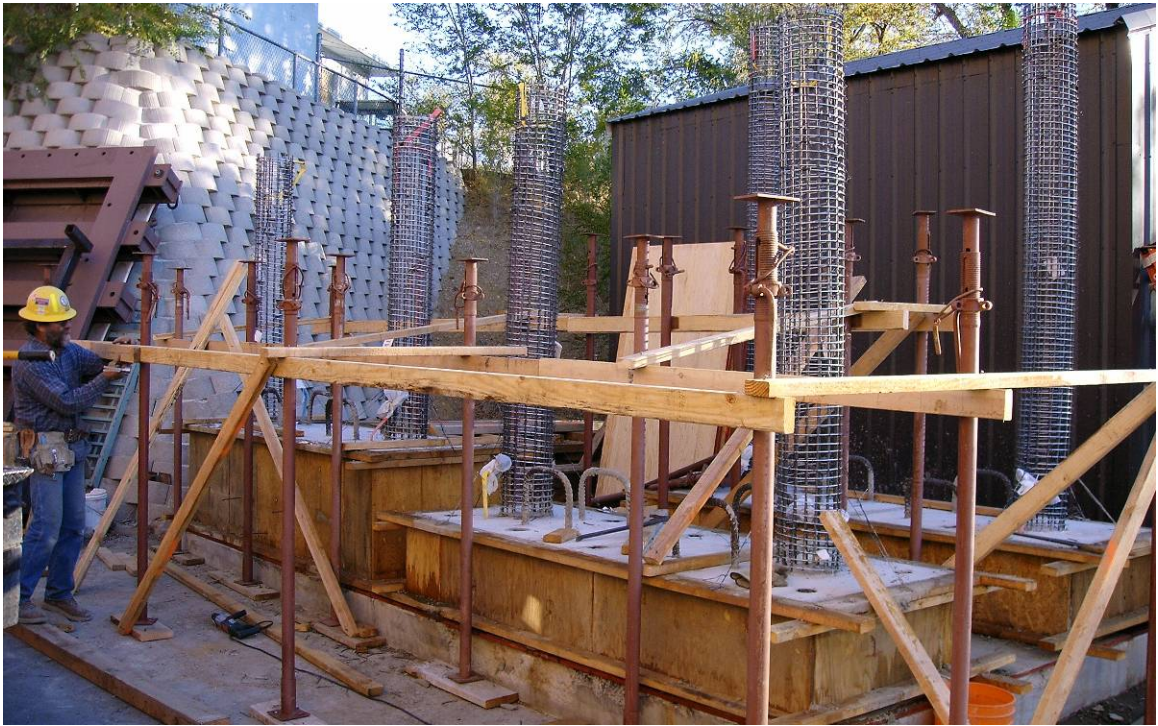
Figure 5-9: Bents after casting of footing concrete and during construction of working platform.
