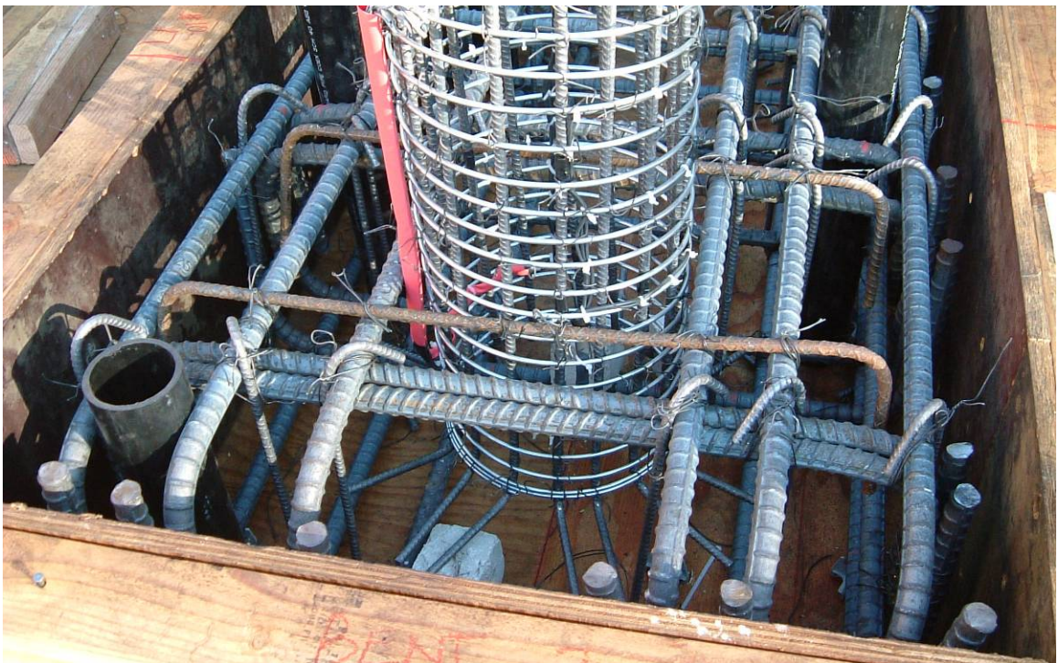
Figure 5-8: Close-up of column cage attachment to footing cage prior to pour of footing concrete.
