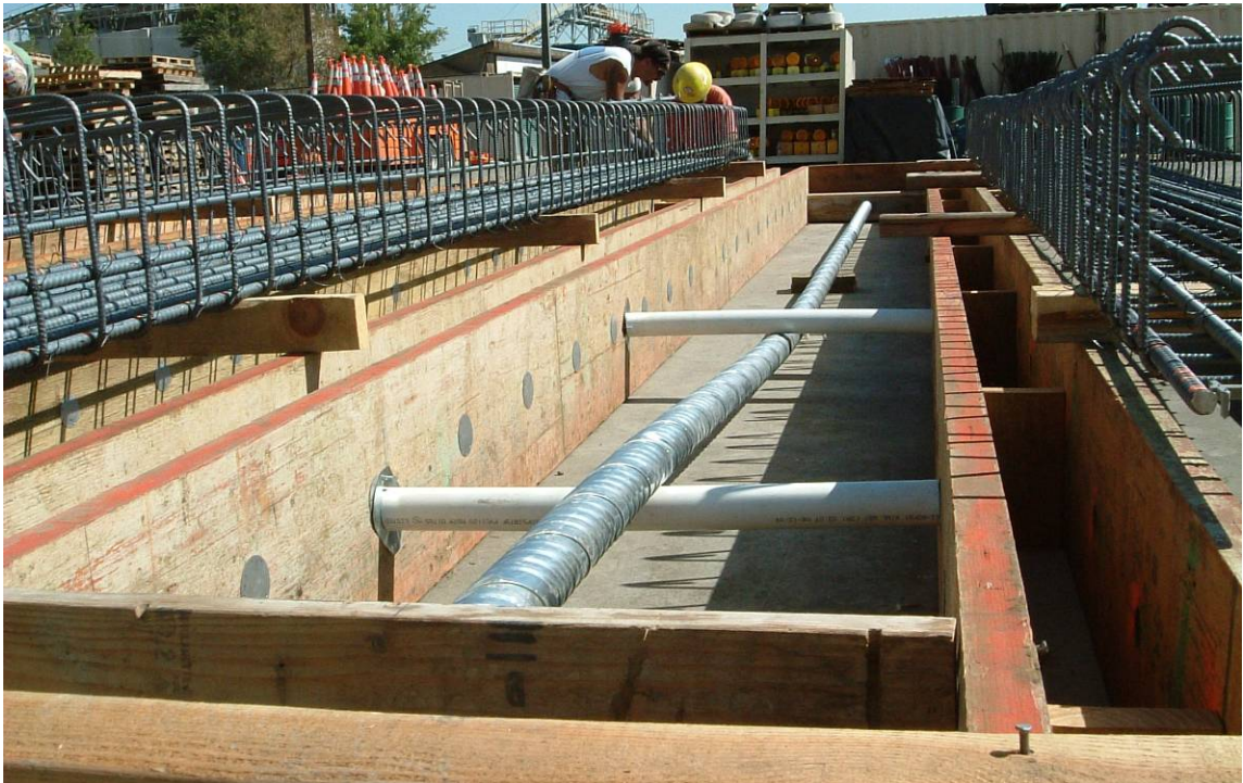
Figure 5-2: Check of longitudinal post-tension duct path prior to placement of reinforcement cages.
