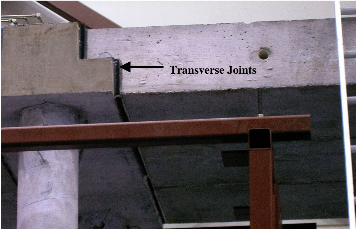
Figure 5-32: Sealing of transverse superstructure joints between bent caps and superstructure beams prior to pouring grout.
