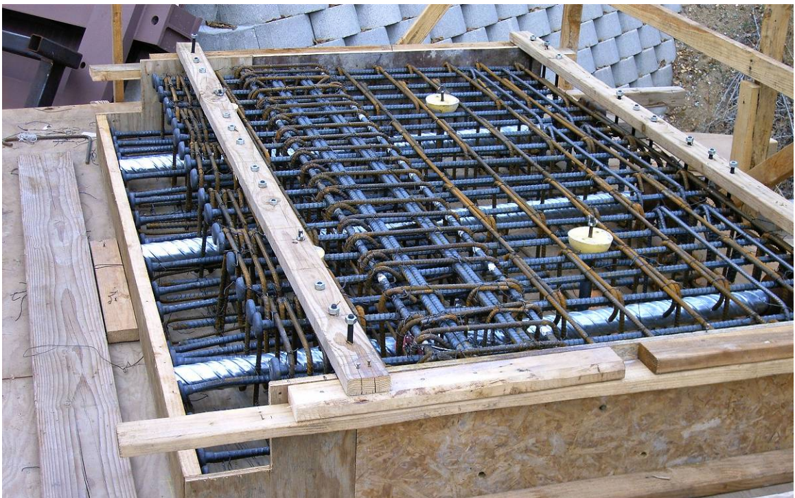
Figure 5-14: Assembly of reinforcement cages and formwork for cantilever cap beams of bents 1 and 3.
