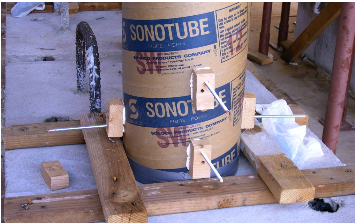
Figure 5-12: Attachment and embedment of curvature rods in columns prior to column concrete pour.
